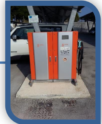
Vehicle-to-Grid Recharging Station
