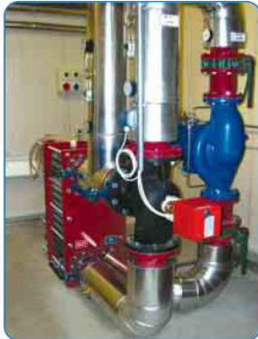
Heat Recovery in centrale termica
