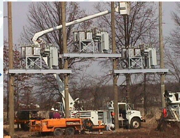
PPP del Delaware Industrial Park: Intellivar Installation – One Phase per Platform. Fonte RSE
