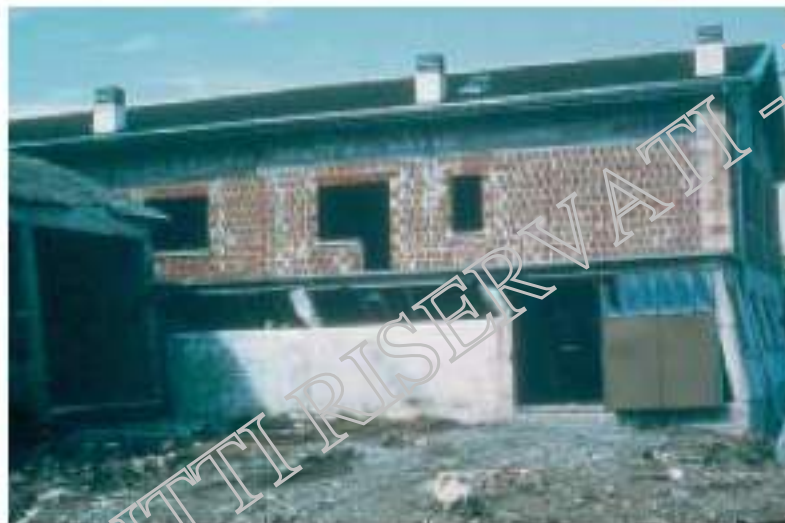
17/1 In this case, inserting parapet walls into a frame led to a short column phenomenon. Owing to the good confinement of the transverse reinforcement, no actual shear failure occurred, but an equally dangerous sway mechanism developed (Friuli, Italy 1976).
