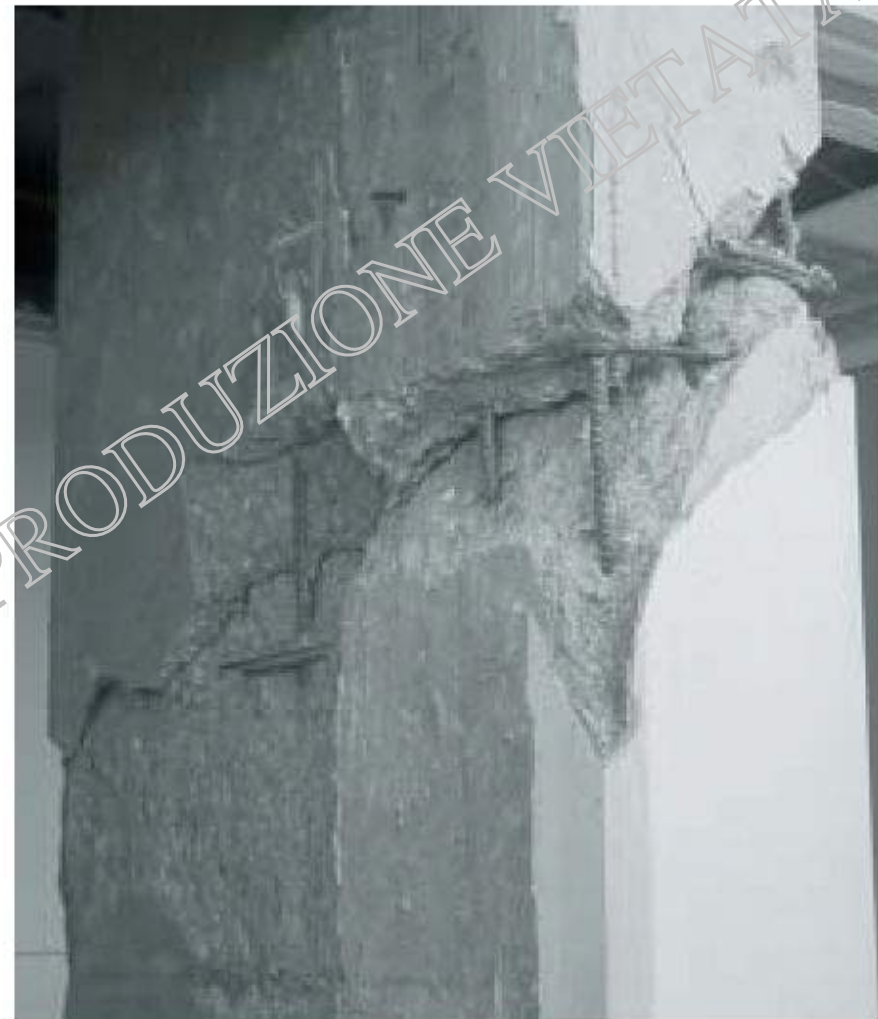
17/3 Better transverse reinforcement in the column (small spaced hoops and ties) would probably have prevented the shear failure. However, the source of the problem lies in the partial infilling of the frame that caused the short column phenomenon (Izmit, Turkey 1999).
