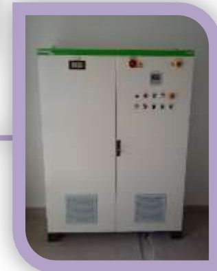
Battery Energy Storage System based on Li Fe PO4 technology
