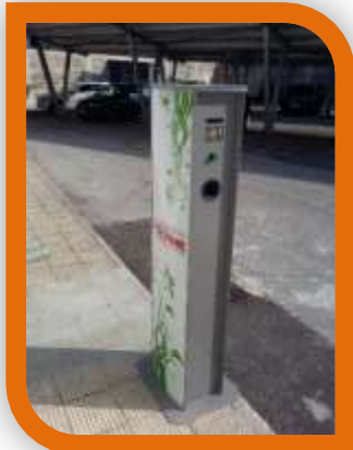
Recharging Station for EVs
